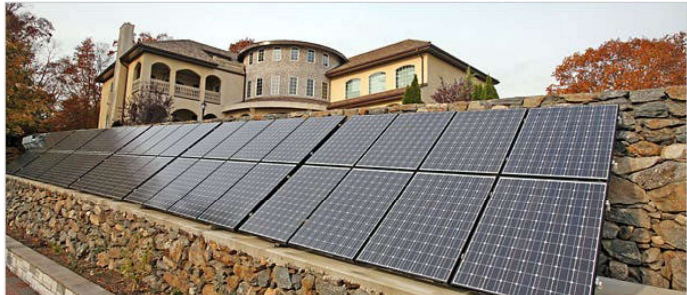
UNDER THE SUN Solar panels are just one of many energy-saving features in Richard and Maryann Ellenbogen's new house. Credit...Suzanne DeChillo/The New York Times
